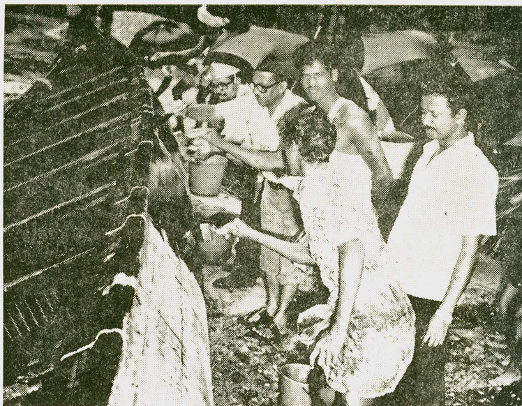
Application of toxic wood preservative on a Thanguvallam (Cochin)
